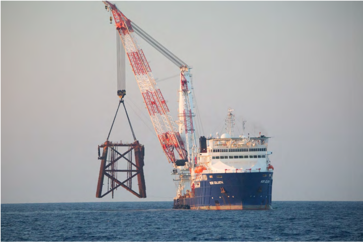
The FGBNMS research team was on hand to observe and photo-document the partial removal of HIA-389A at East Flower Garden Bank. The majority of the structure, from 65 ft to the seafloor at around 400ft depth, is still in place. Photo: G.P. Schmahl/NOAA
